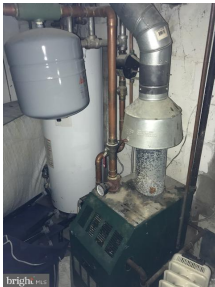
Utility Room-Gas Furnace
