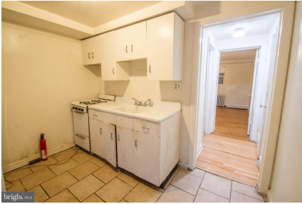
This is the basement unit - now damaged by water
