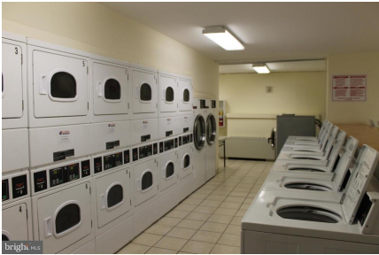
On-Site Laundry Facilities
