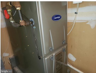
Newer gas furnace
